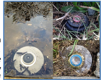
Irrigation cross connection
