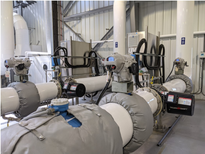
UV Disinfection System
