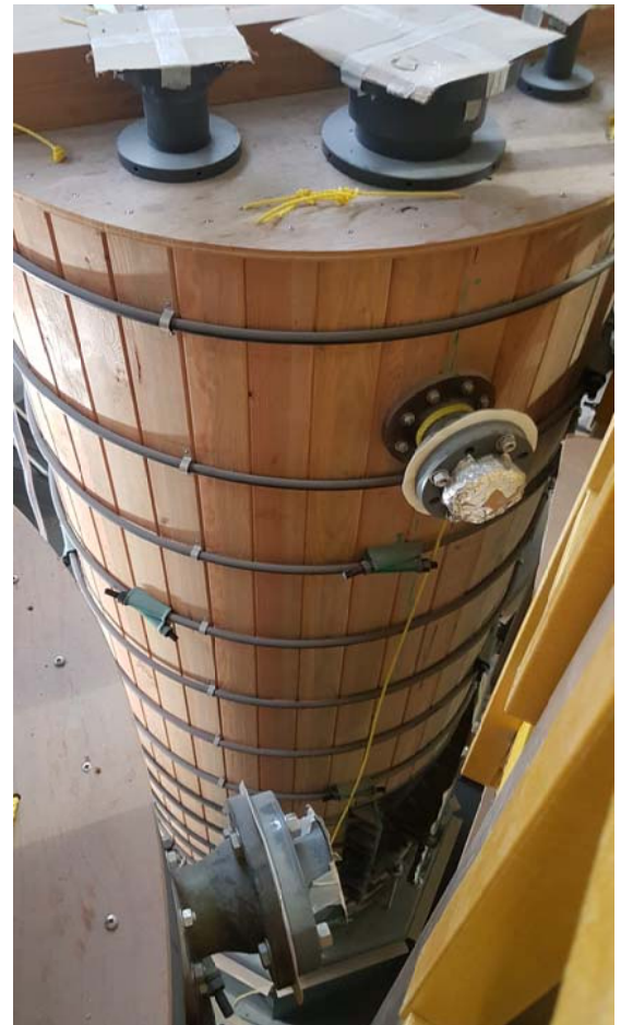
Sodium Hypochlorite tank
