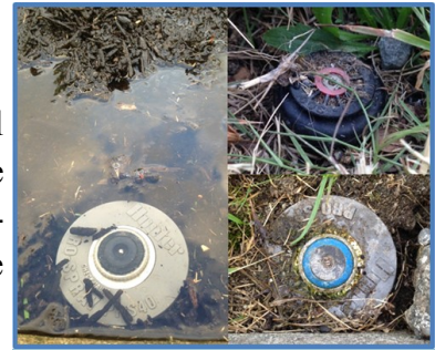
Irrigation cross connection
