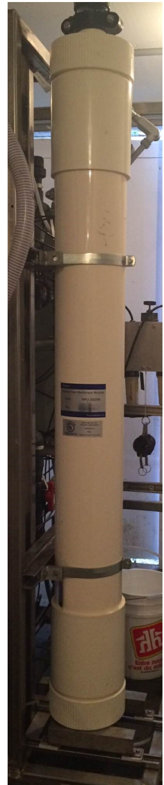
Pilot Plant—UF membrane system
