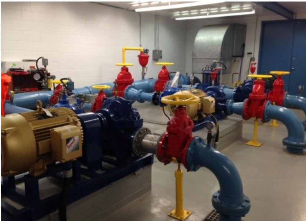
Springwood Pump Station
