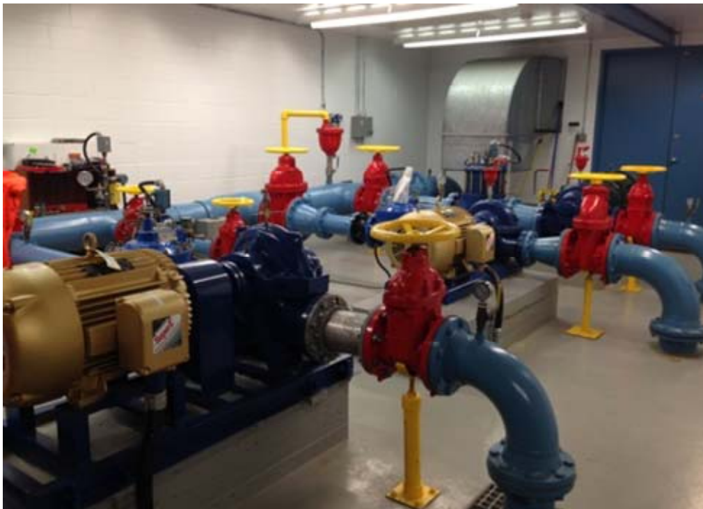
Springwood Pump Station
