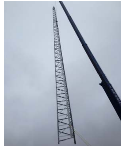
New communication tower
