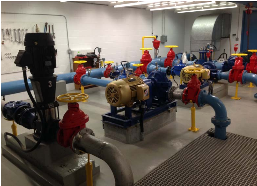
Springwood Pump Station
